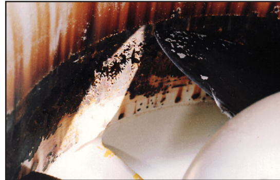
Cavitation and erosion of bell housing
