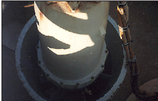
Three pumps were experiencing this failure
